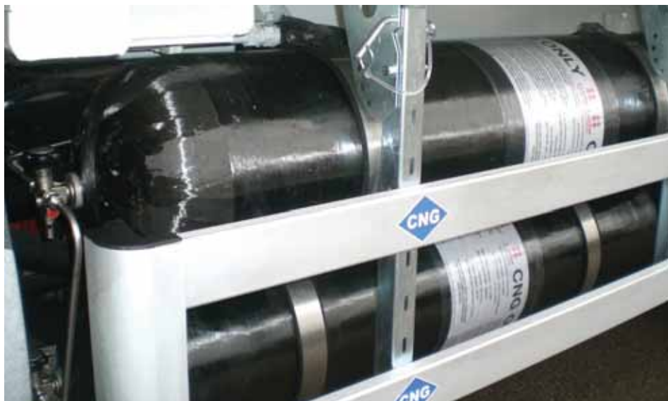
Typical installation for composite CNG cylinders
