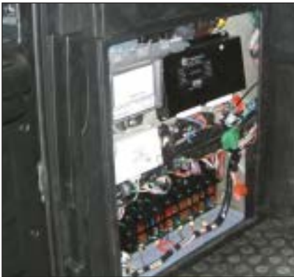
In cab - the Elite 2's solid state electrics are conveniently housed for ease of access.
